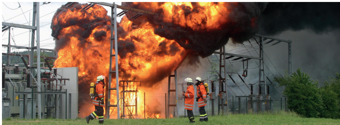
Transformer fire at a nonprotected site
